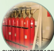
CHEMICAL STORAGE BATTERY CHARGING ROOMS
